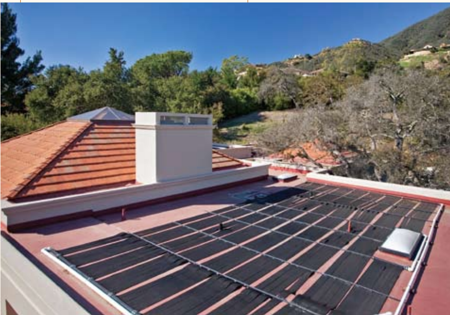
Above: A recently installed solar pool heater is hidden from view on this flat roof.
